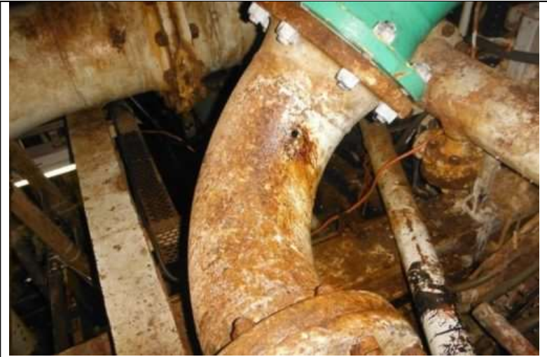
Pipework - Applied to all components of pipework suffering from wall loss.
