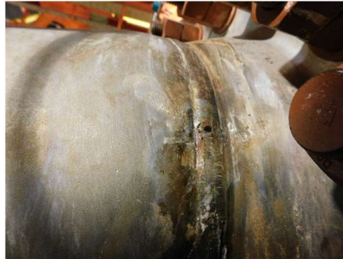
Initial condition of weld
