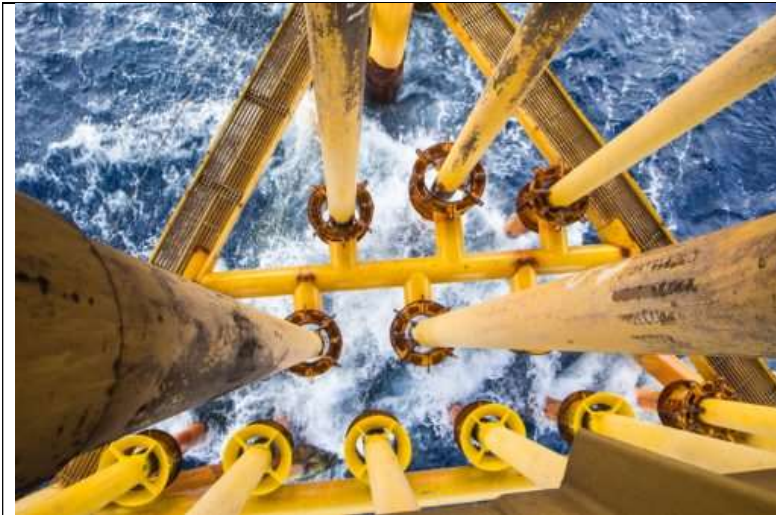
Caissons and Risers - Applied to caissons and risers above, below and within the splash zone.
